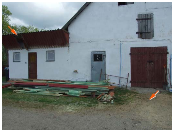
Fot. 5. The hole in the roof and the place where the meteorite was found (marked by arrows)
