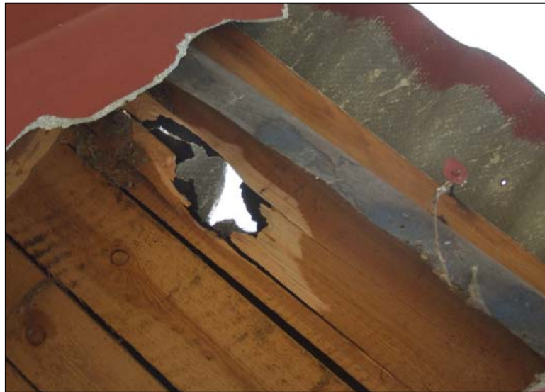
Fot. 3. The hole in the roof of the shed – the first place of contact between the Soltmany meteorite and solid Earth
